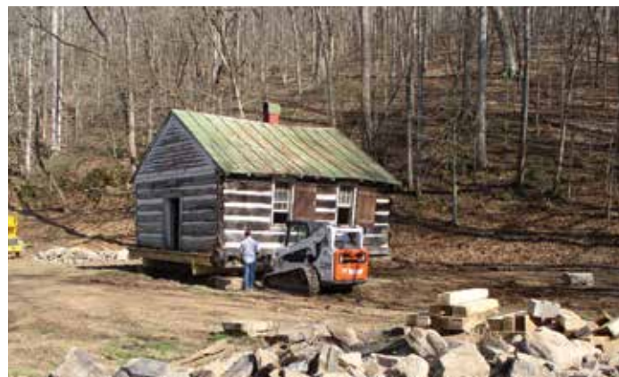
Will and Tommy Harris prepare the Hamilton Schoolhouse for a stone foundation.
