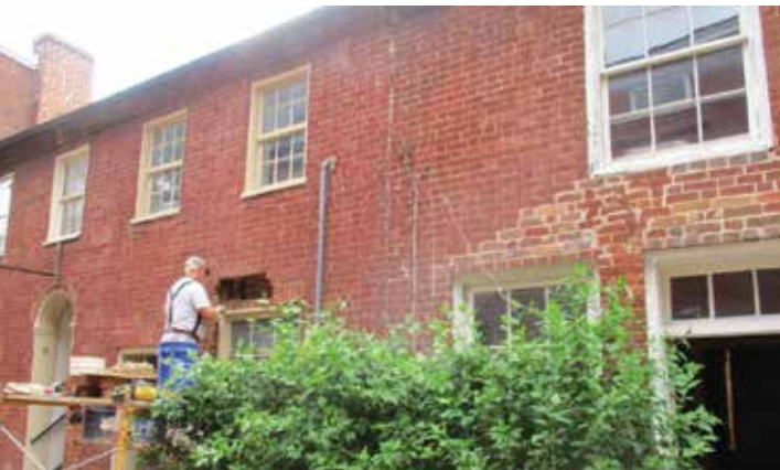
May - HLF façade grant supports re-pointing and other repairs to Lawyer's Row building designed by Thomas U. Walter.
