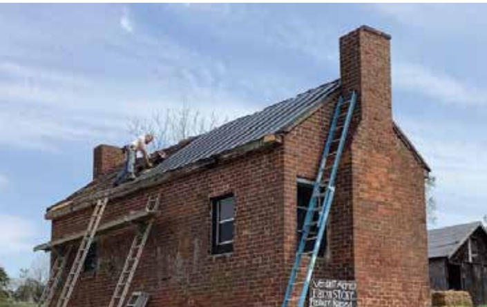
Thanks to an HLF grant through the Lyle-Simpson Preservation Fund, the former slave quarters at Verdant Acres now has a new roof.
